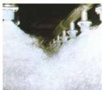
Tower desulfurization in power station
